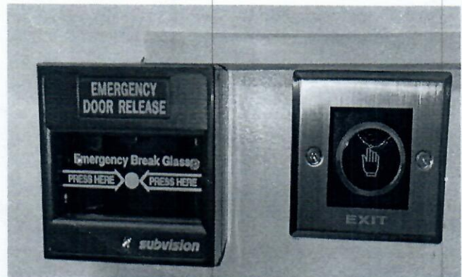
Sensor Exit dan Emergency Exit
