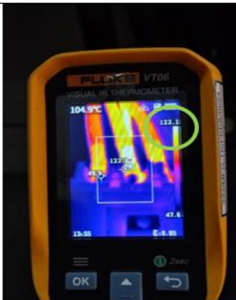
Incoming MCCB Chiller 6B (up to 122°C)
