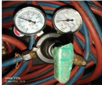
Regulator Oksigen/Nitrogen Existing
