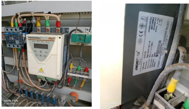
3. Inverter motor pompa chiller AHU 8B
