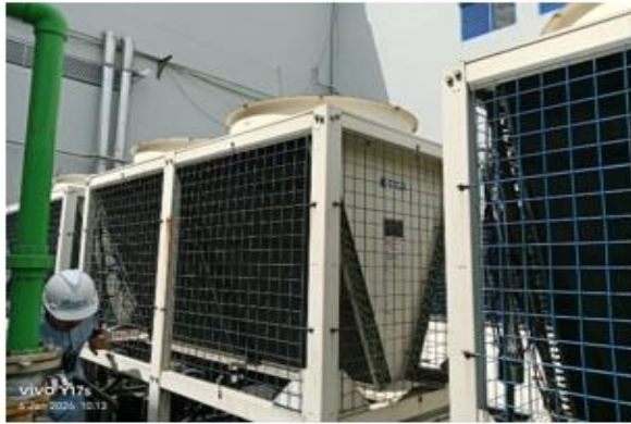
Chiller 2 HMI 1 6A
